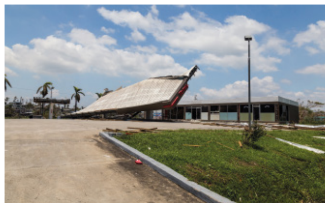
Destruction of petrol station caused by Tropical Cyclone Winston, Island Viti Levu, Fiji.
