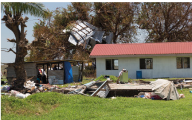
The effects of Tropical Cyclone Winston, December 2016.
